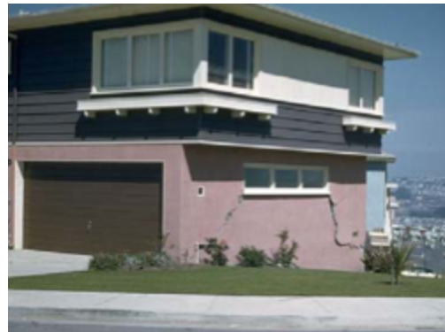
Cracks in a masonry are a sign of danger.
