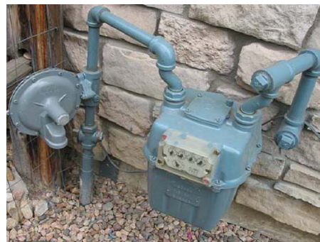
Natural gas shut off valve next to meter
