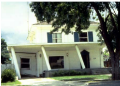
Leaning porch after an earthquake
