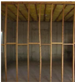
Deformed studs in open bearing walls
