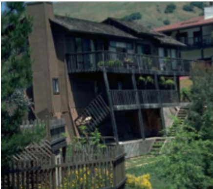
The entire wall near the chimney is out of plumb.
